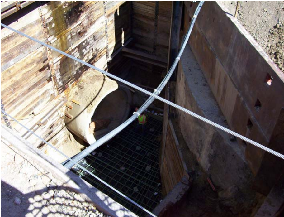
Photo 2: Construction of Campus Drive structure (S-1 in plan set). Contractor shall tap into this structure as detailed in the Special Provisions. The shoring system shown in the photo, or portions of the shoring system were most likely left in place.
