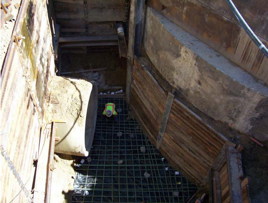
Photo 1: Construction of Campus Drive structure (S-1 in plan set). Contractor shall tap into this structure as detailed in the Special Provisions. The shoring system shown in the photo, or portions of the shoring system were most likely left in place.
