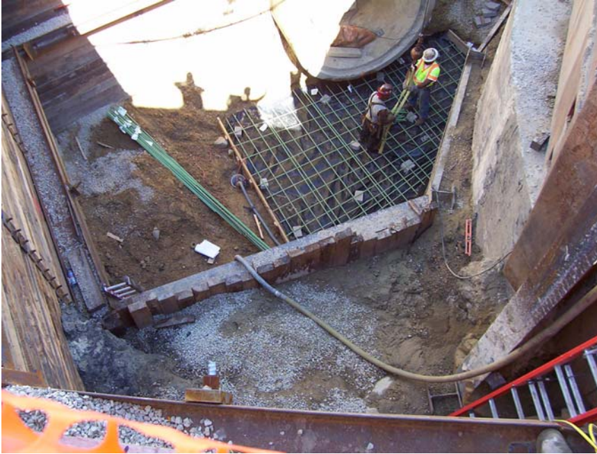
Photo 3: Construction of Campus Drive structure (S-1) in plan set. Contractor shall tap into this structure as detailed in the Special Provisions. The shoring system shown in the photo, or portions of the shoring system were most likely left in place. The structure wall to be tapped is shown on the left side of the photo.
