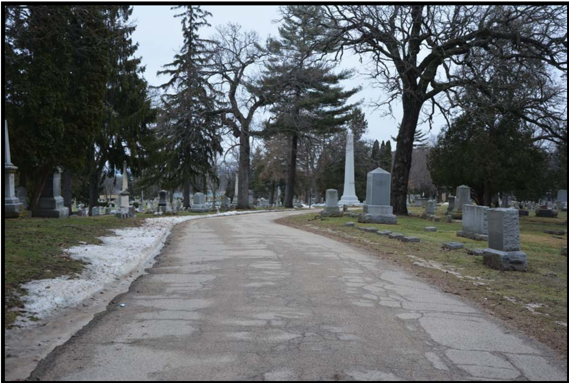
Figure Nineteen: Example of roadway conditions and previous repairs.
