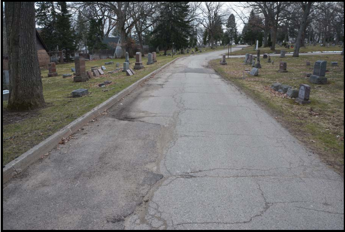
Figure Eighteen: Example of roadway conditions and previous repairs.
