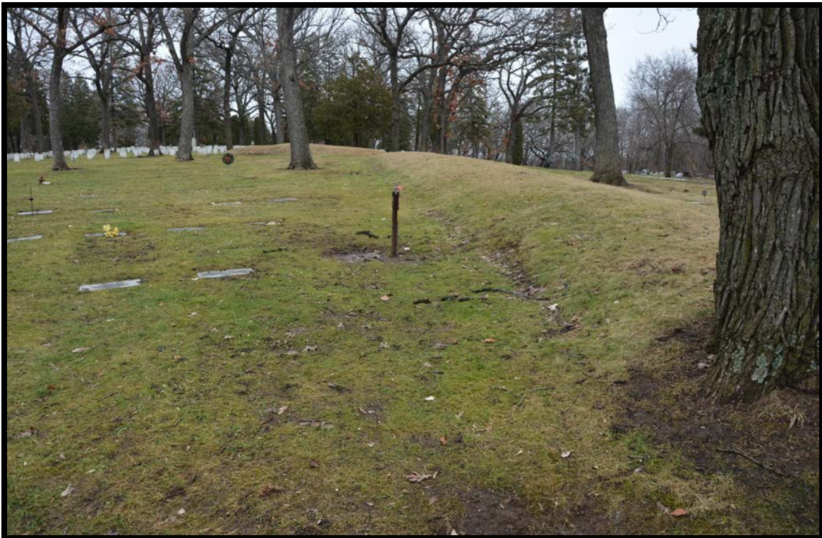
Figure Seven: Existing standpipe (center of image) to be removed at DA-134.
