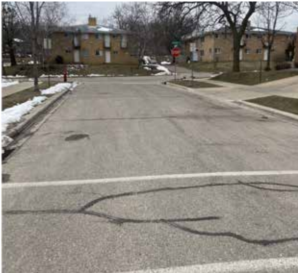
Mike McKinney Ct (tarred cracking, fading cross line paint)
