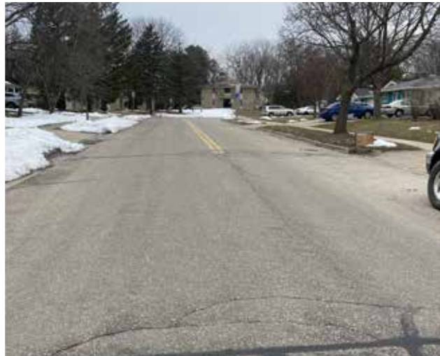
Crescent Road (cracking, and generally fair)
