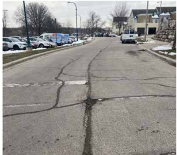
Revival Ridge (cracking, crumbling along center, fading marking paint)
