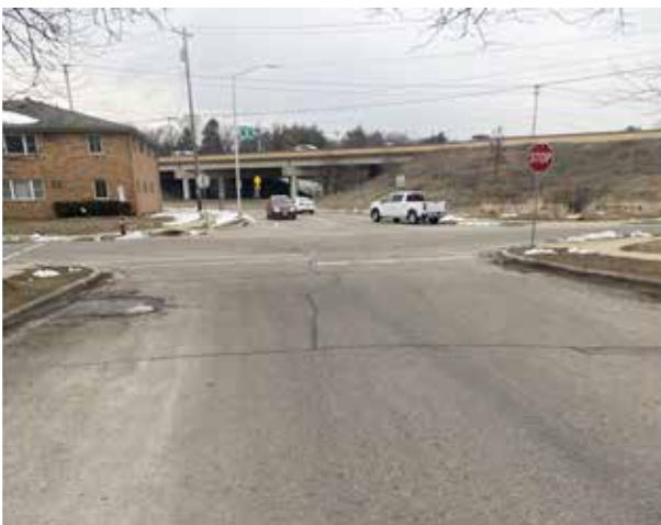
Thurston Lane (tarred cracks, fading marking paint, fair condition)
