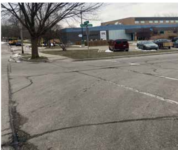
Jenewein Road (tarred cracks, crumbling along gutters, fading line paint)
