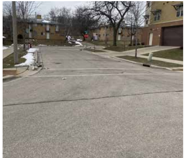
Mike McKinney Ct (tarred cracking, fading cross line paint)
