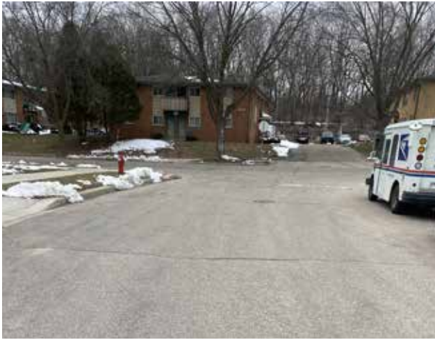
Dunns Marsh Terrace (minor cracking, fading road marking, fair condition )
