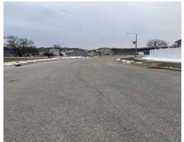
Percy Julian Way (minor cracking, relatively fair)
