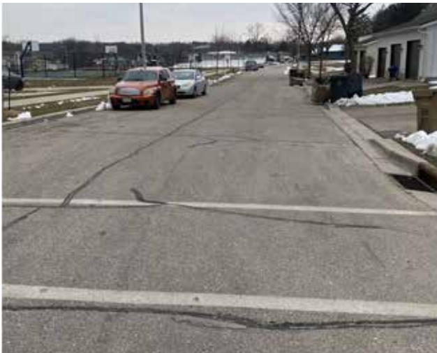
Gene Parks Place (cracking, uneven surface and settling)
