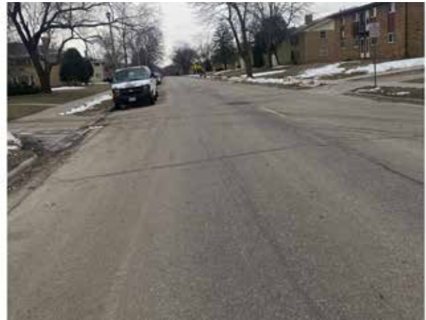
Allied Dr (cracking, some minor potholes toward the end)
