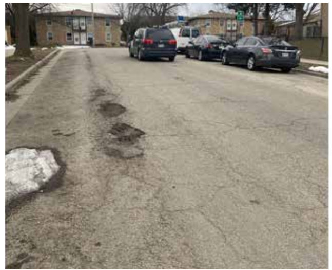
Jenewein Road (cracking, potholes, aggregate showing)
