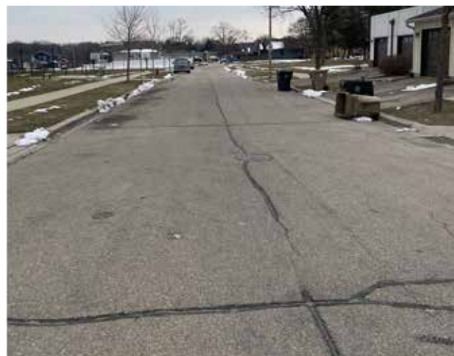
Gene Parks Place (cracking, uneven surface)
