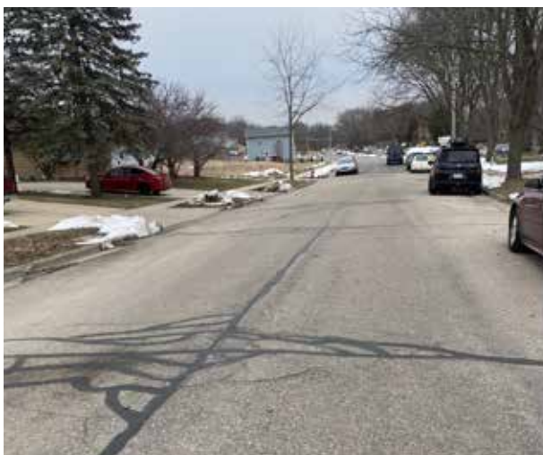
Crescent Road (cracking and uneven surface)
