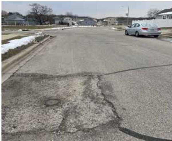
Percy Julian Way (cracking, poor tarred finishes in a section, fading cross line paint)
