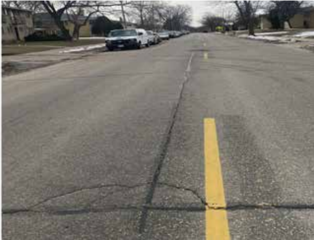
Allied Dr (cracking, some minor potholes toward the end)
