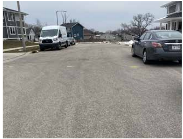
Dunns Marsh Terrace (minor cracking, fading marking)
