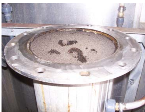
Photo 7: Dual Media After Testing – Sand at Surface
