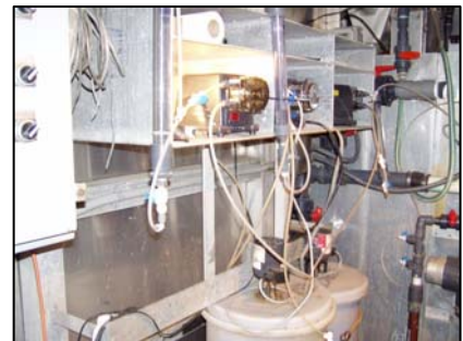
Photo 5: Filters 1, 2, and 3 Chemical Feed Pumps and Tanks
