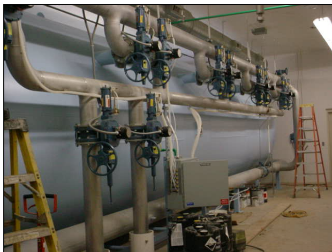
Photo 12: Horizontal Pressure Filter
