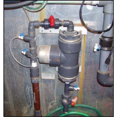
Photo 4: Pressure Aeration Unit - Atomerator
