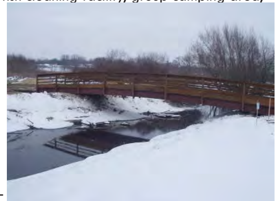
Photo: Bridge in Nine Springs E-Way near Baxter Park, joint County and City project, photo courtesy of Dane County Parks
