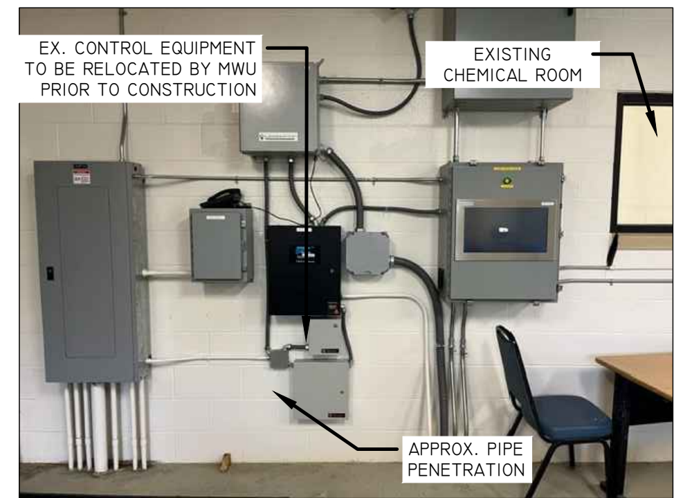
EXISTING CONTROL EQUIPMENT FACING SOUTHWEST
