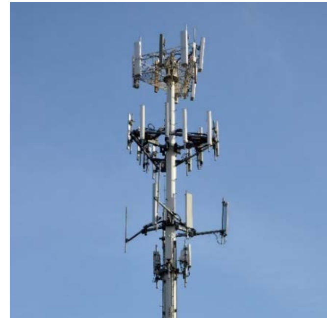
Typical large cellular antenna Photo credit: Joe Ravi via Wikimedia Commons
