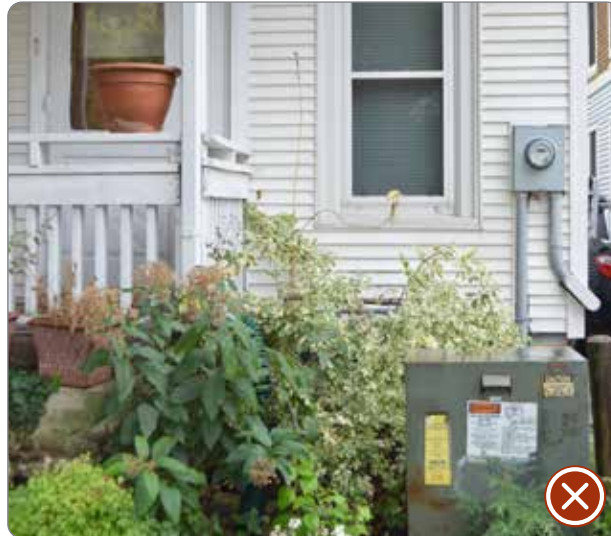
Figure 82: Utilities at the front of a building, in this placement, it should be screened with fencing or landscaping (41.25.7.a.2).
