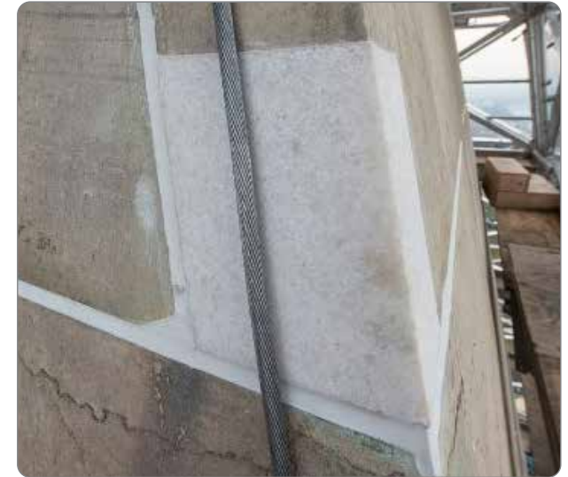
Figure 34: Example of a dutchman repair.
