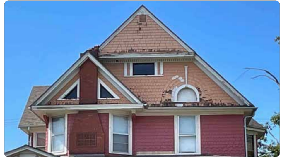
Figure 17: Example of wood siding needing to be re-painted on a residence that is otherwise in good condition (41.23.3.b.1).
