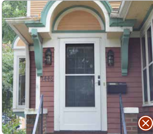
Figure 106: Incompatible storm door, new storm doors need to be full light (41.26.5.d.1).
