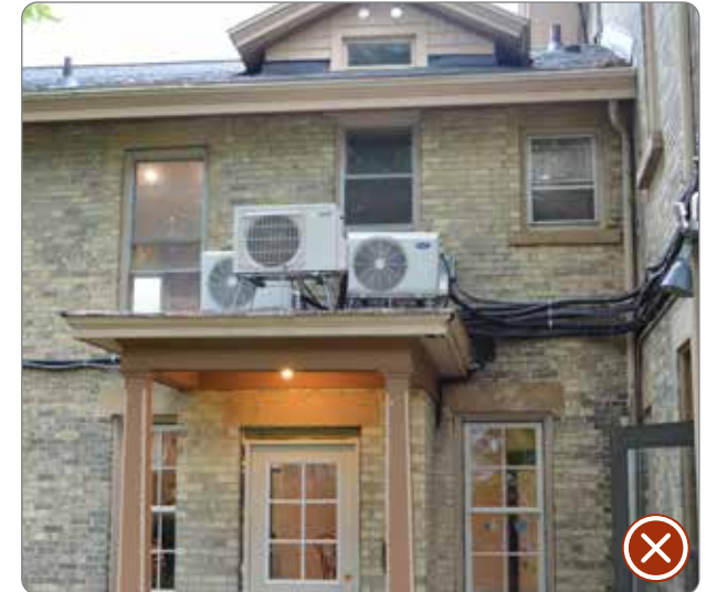
Figure 83: Placement of mechanical equipment that is highly visible from the public right-of-way (41.25.7.a.3).
