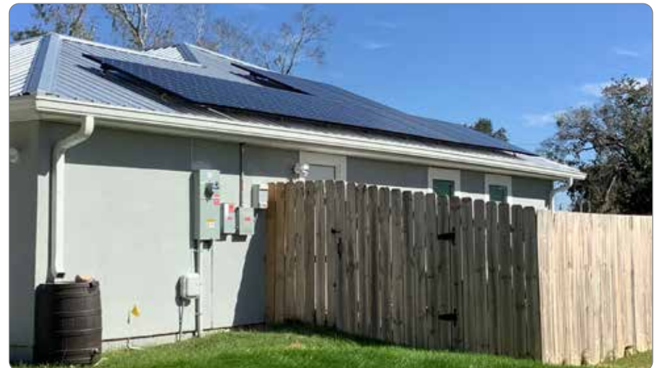
Figure 141: Solar panel installation minimally visible from the public right-of-way (41.27.7.b.2).
