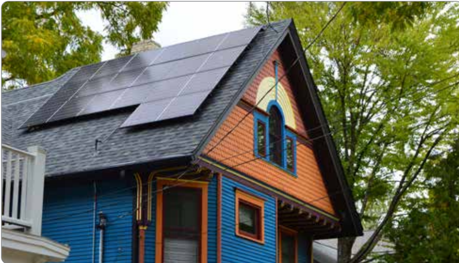
Figure 84: Example of solar panel roof installation (41.25. 7.b).
