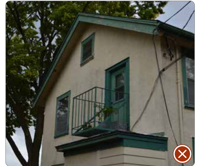
Figure 114: Incompatible balcony addition on the side of a building (41.26.6.b).
