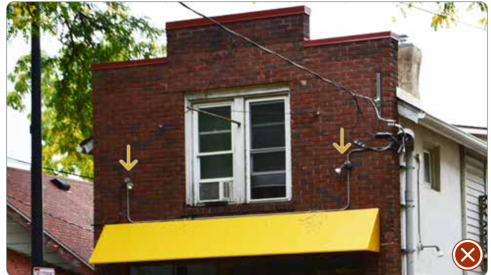
Figure 143: Example of obtrusive security lighting and exposed conduit (41.27.7.c.2-3).
