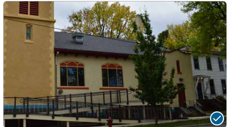
Figure 49: Compatible accessibility ramp constructed on side of historic public building at 504 S Breatly Street (41.25.1.d.2).
