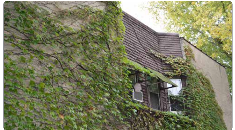
Figure 21: Growing vegetation that should be removed (41.23.3.d.2).
