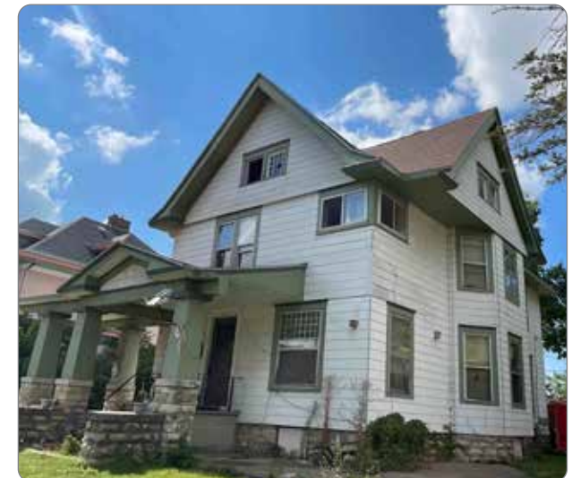
Figure 11: Low Integrity Building.
