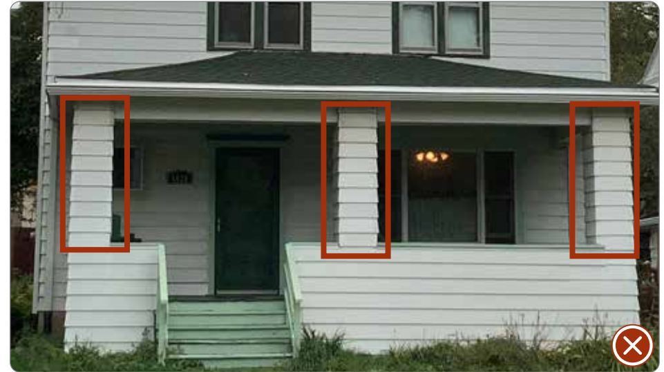
Figure 54: Incompatible wrapped wood columns (41.25.3.b.4).
