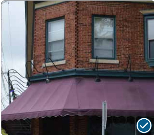
Figure 118: Commercial decorative lighting (41.26.7.c.1).
