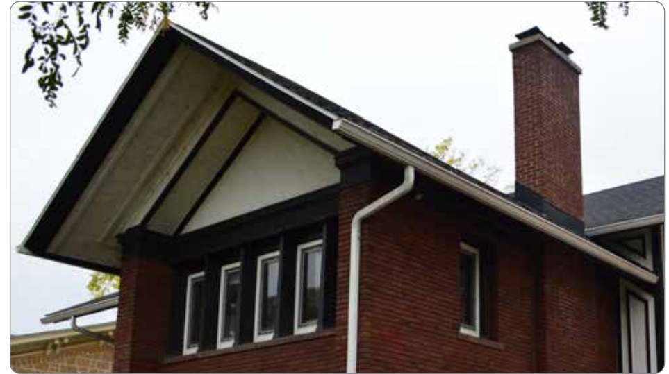
Figure 22: Example of a maintained roof system at 514 N Carroll Street (41.23.4.a.1).
