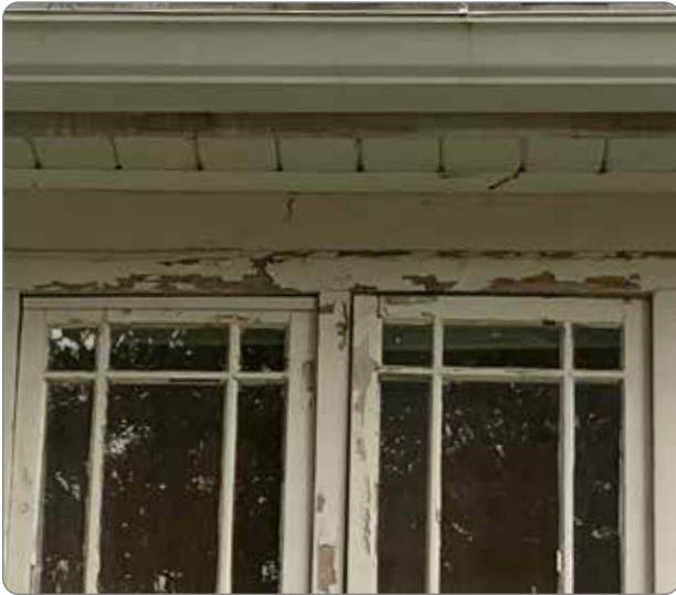
Figure 39: Wood features requiring repair (41.24.2.b.1).
