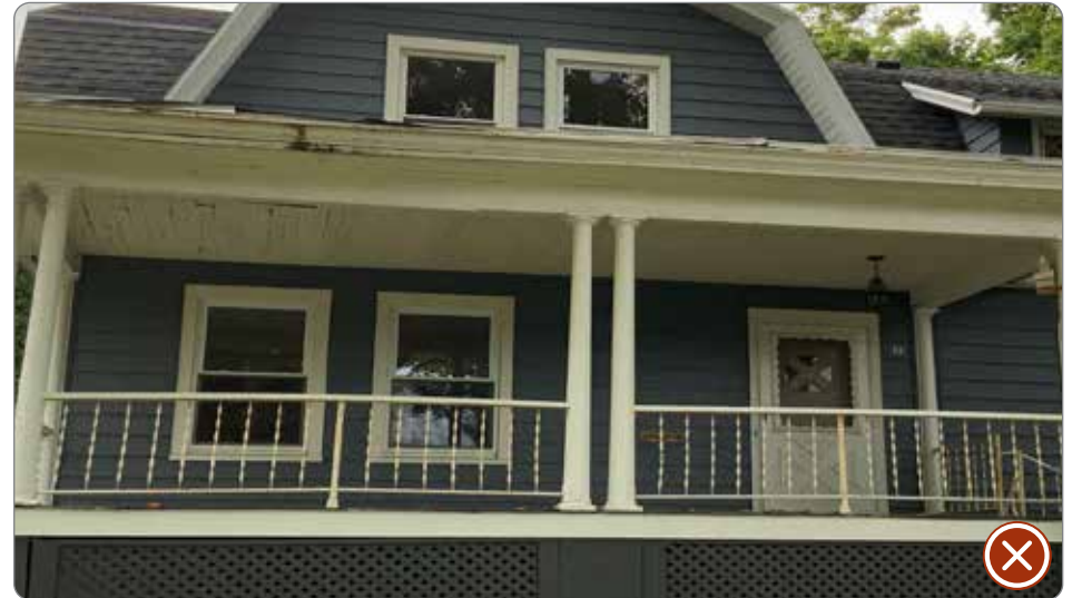
Figure 57: Incompatible substitute metal replacement (41.25.3.c.1).
