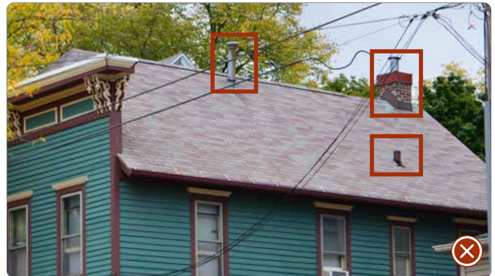
Figure 60: Example of ridge vent and a prohibited electric vent visible from the developed public right-of-way (41.25.4.e).
