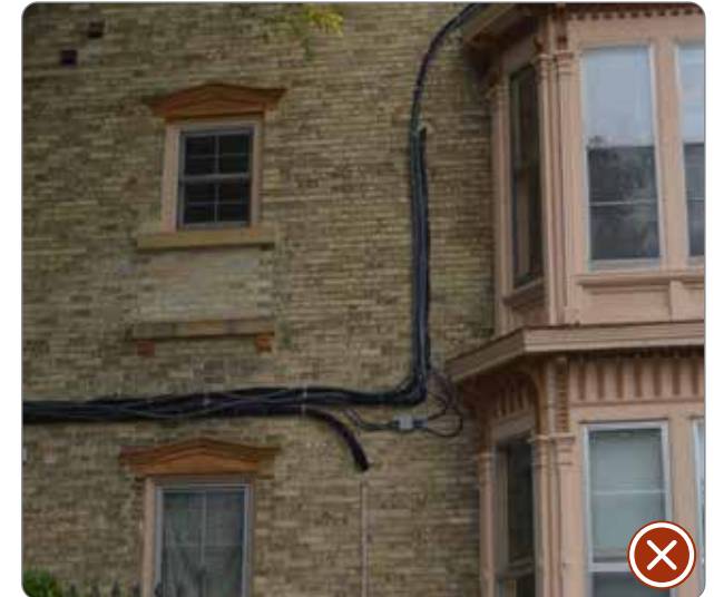
Figure 120: Exterior mounted conduit on historic building elevation (41.26.7.c.3).
