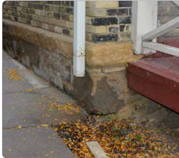
Figure 13: Improper drainage gutter system resulting in deterioration of foundation walls (41.23.2.a.1).
