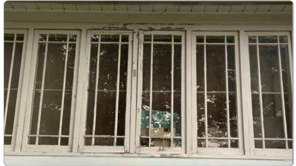
Figure 41: Example of windows in need of repair (41.24.5).
