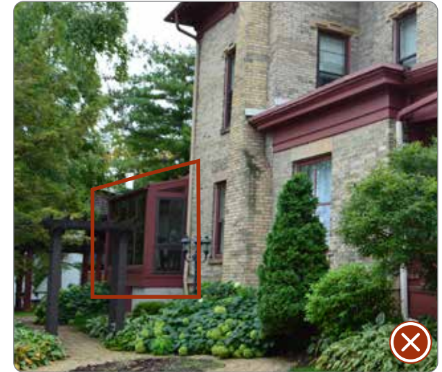
Figure 104: Addition windows that are incompatible with historic building (41.26.5.a.1-2).
