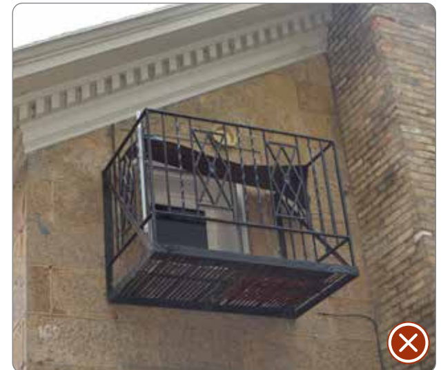
Figure 115: Incompatible balcony addition on front elevation (41.26.6.b).
