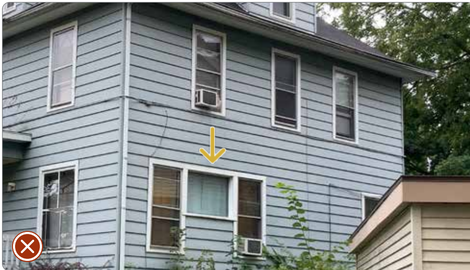
Figure 61: Incompatible window opening, visible from the right-of-way, not in keeping with existing visual qualities (41.25.5.a.1).
