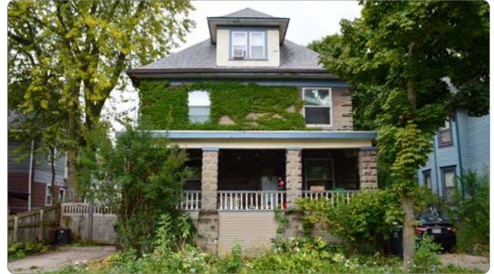
Figure 20: Vegetation on a masonry building can damage the masonry and mortar (41.23.3.d.2).
