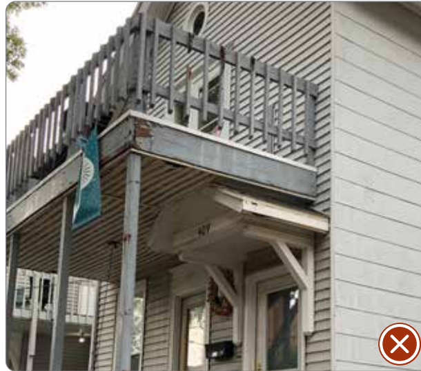
Figure 113: Incompatible balcony addition with out of character railing balusters and the deck cutting off the top of the gabled portico over the door (41.26.6.b).
