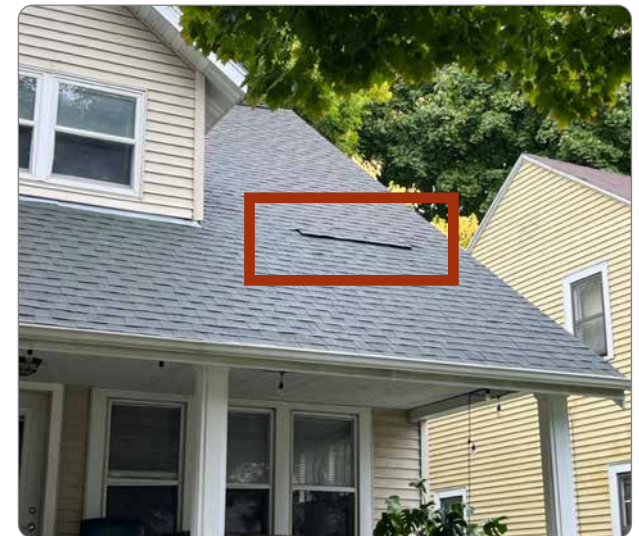
Figure 99: Minimally visible roof vent (41.26.4.e.1).
