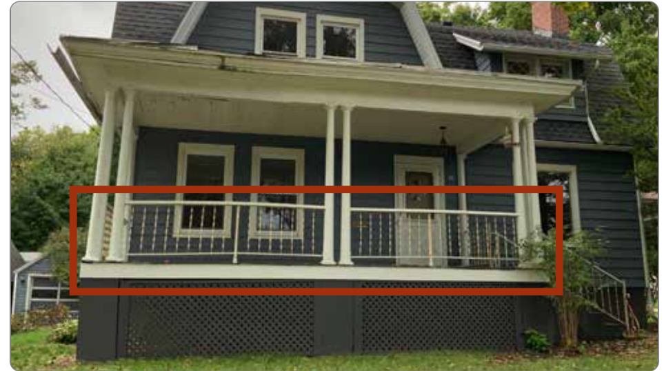
Figure 73: Example of a replacement railing that is out of character for the style house (41.25. 6.a.1).
