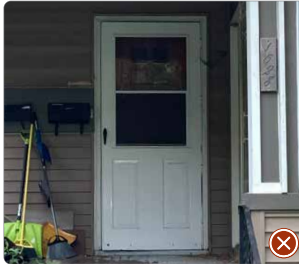
Figure 70: Example of an incompatible storm door. New storm doors need to be full light (41.25.5.d.3).
