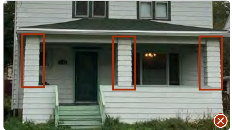
Figure 54: Incompatible wrapped wood columns (41.25.3.b.4).
