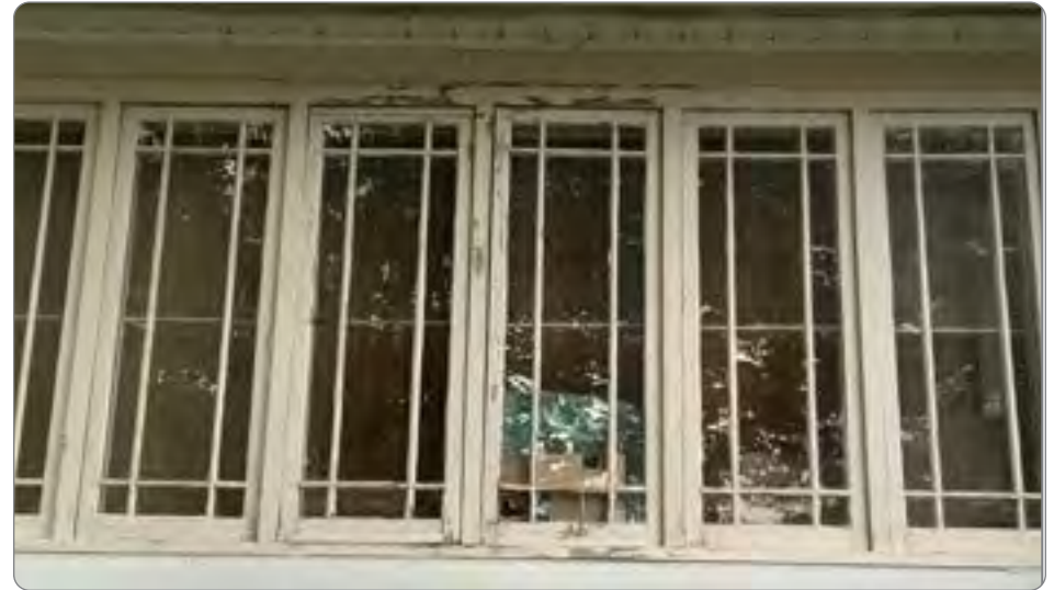
Figure 41: Example of windows in need of repair (41.24.5).
