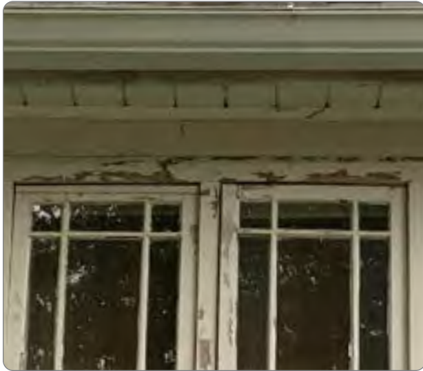
Figure 39: Wood features requiring repair (41.24.2.b.1).
