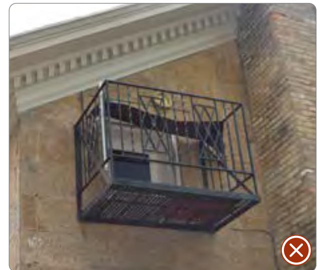
Figure 115: Incompatible balcony addition on front elevation (41.26.6.b).
