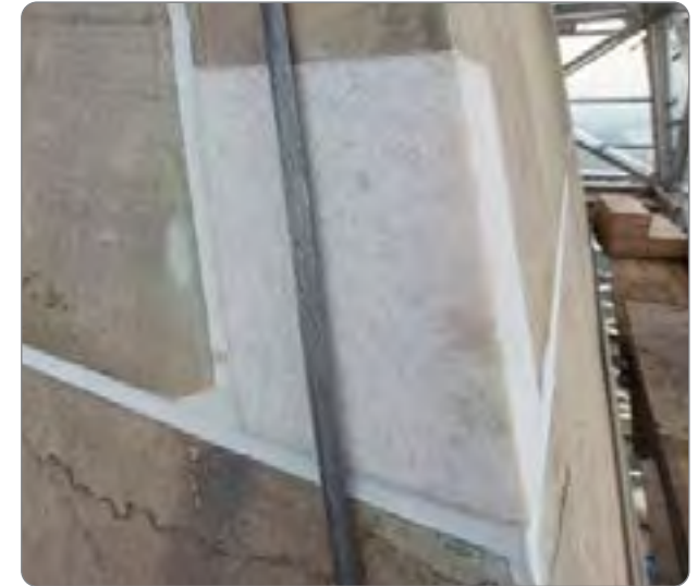
Figure 34: Example of a dutchman repair.
