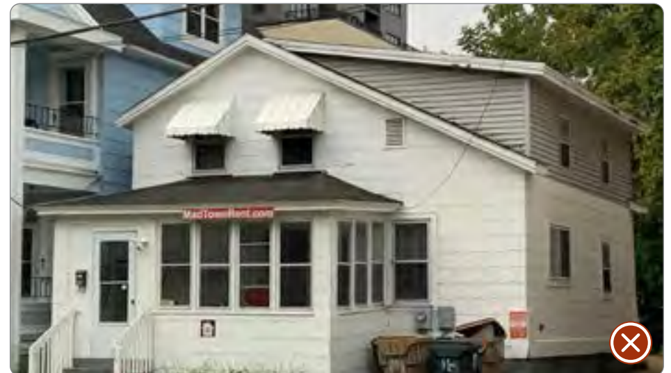
Figure 101: Incompatible dormer addition to residence (41.26.4.f.1-4).
