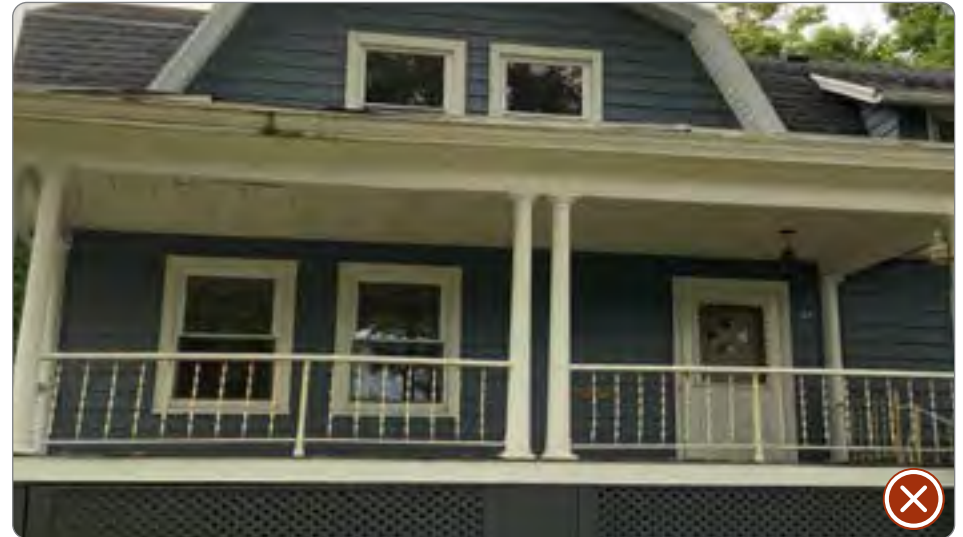
Figure 57: Incompatible substitute metal replacement (41.25.3.c.1).
