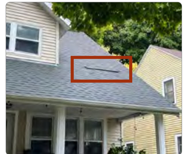
Figure 99: Minimally visible roof vent (41.26.4.e.1).
