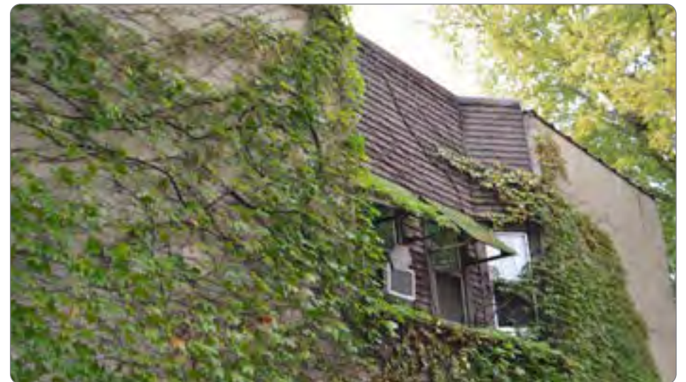
Figure 21: Growing vegetation that should be removed (41.23.3.d.2).
