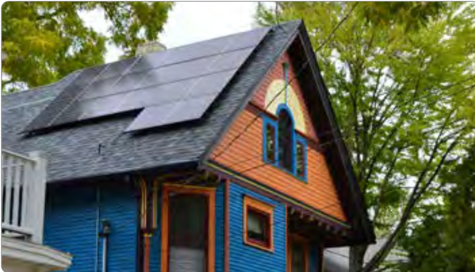
Figure 84: Example of solar panel roof installation (41.25. 7.b).
