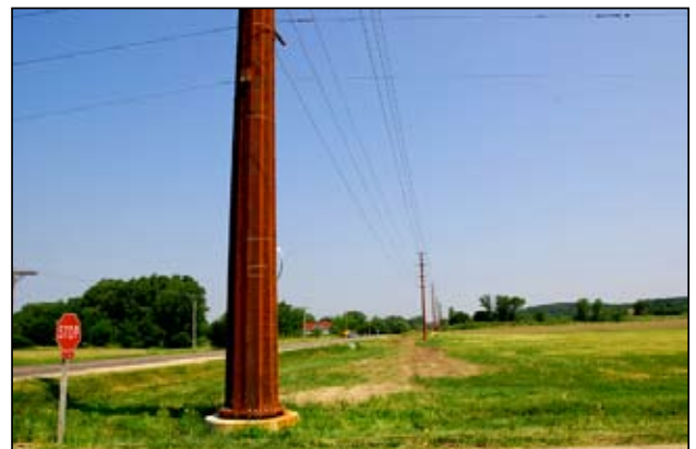
Overhead electric transmission lines along Reiner Road
