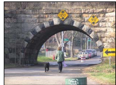
The railroad viaduct at Bram-Koster poses unsafe conditions for pedestrians because of its narrow width.
