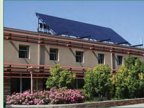
Solar panel example
