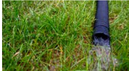
Residential sump pump discharging water from end of flexible black hose.
