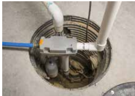
Standard sump "crock" where the water from the perimeter is piped below the floor.
