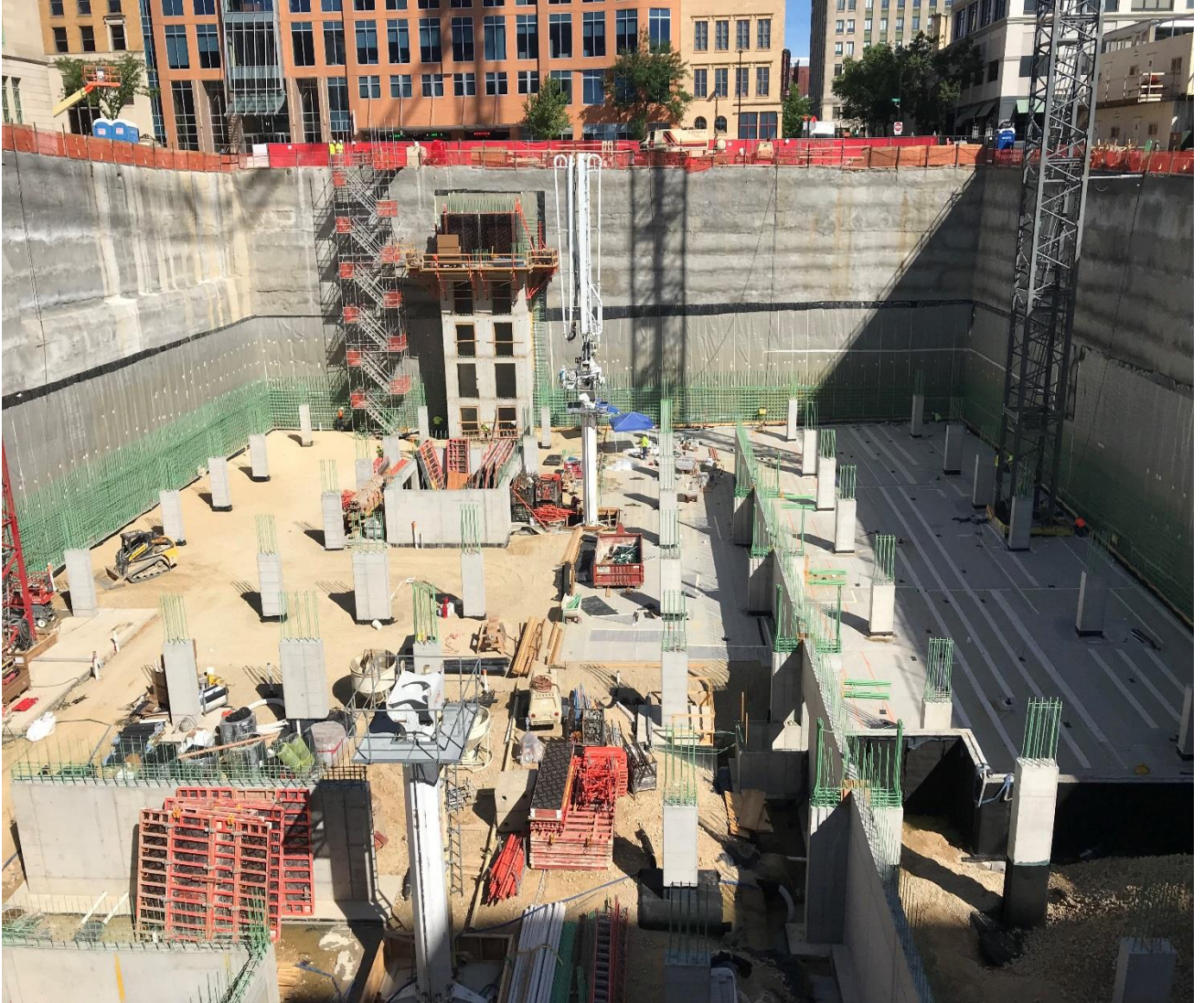
An image of the progress to date looking to the north to Doty Street and Block 89.
