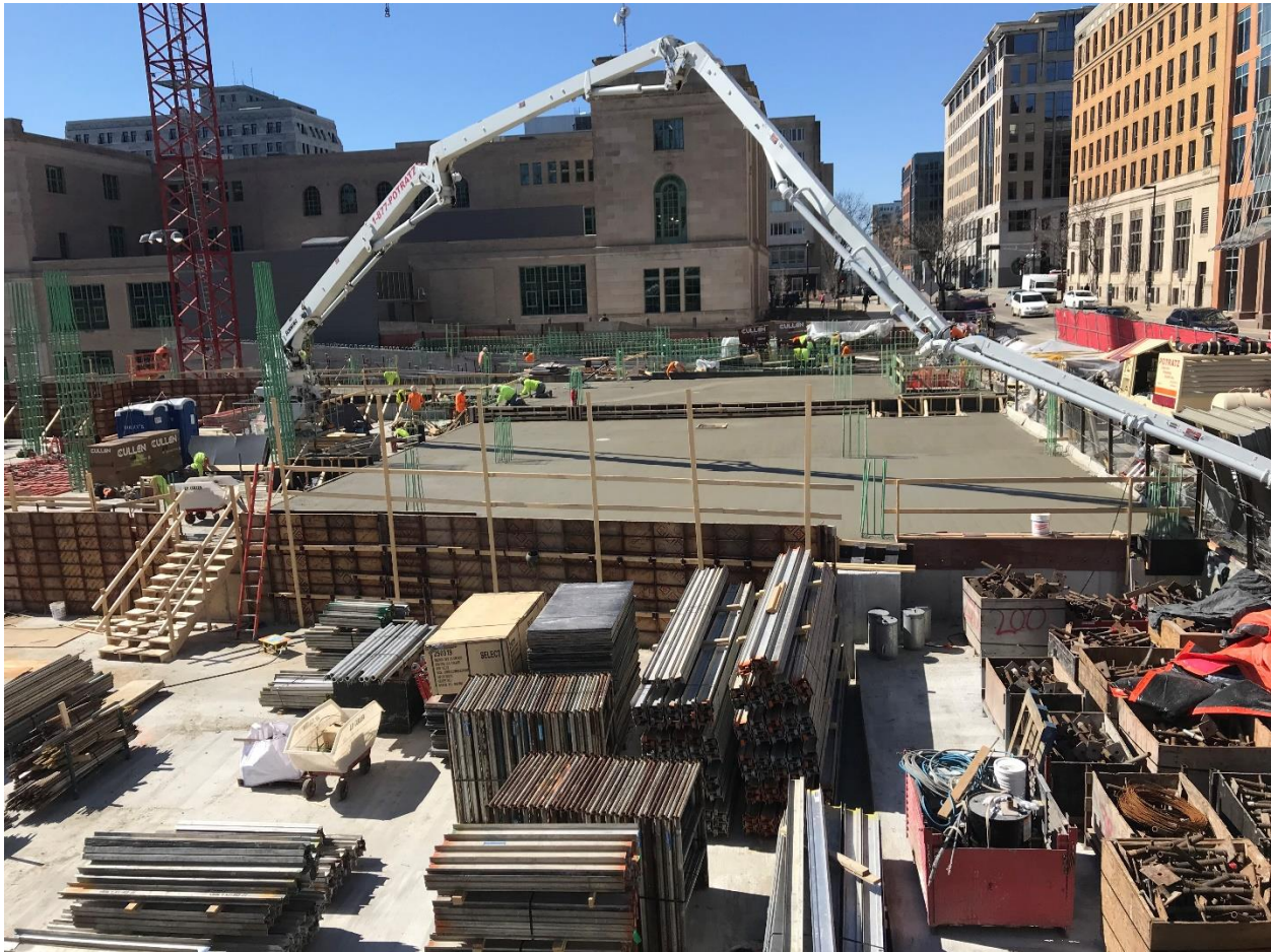
An image of a concrete deck pour along East Doty Street looking west towards the Madison Municipal Building.
