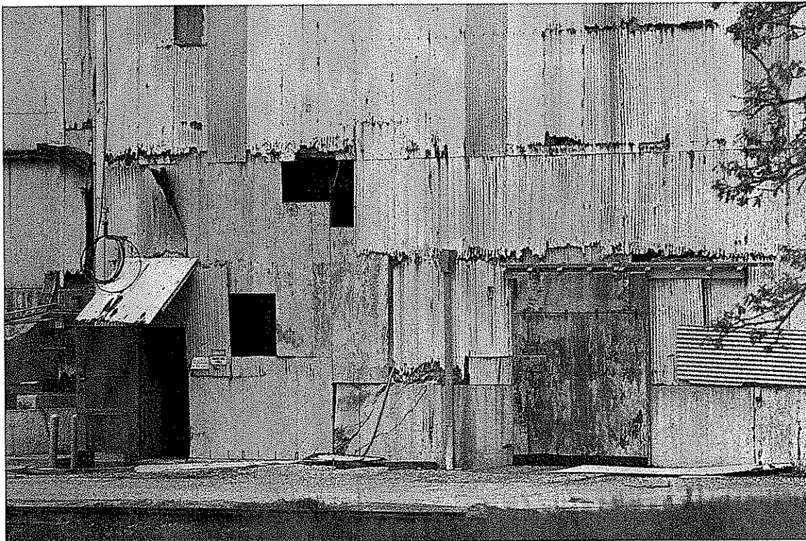
Condition of walls and doors on exterior of granulation building, May 2008
