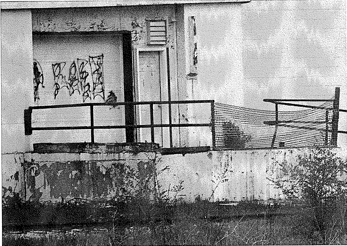
Broken rail on exterior of Shop Building, May 2008
