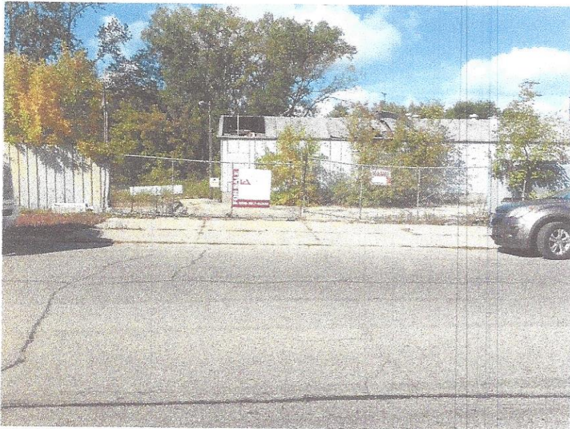
Front entry curb cut, fenced gated entry, metal building to demo with damaged roof
