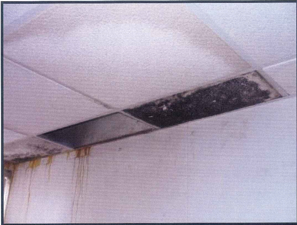
Water damage due to leaking roof
