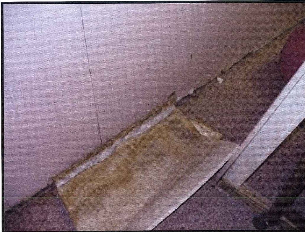
Additional water damage
