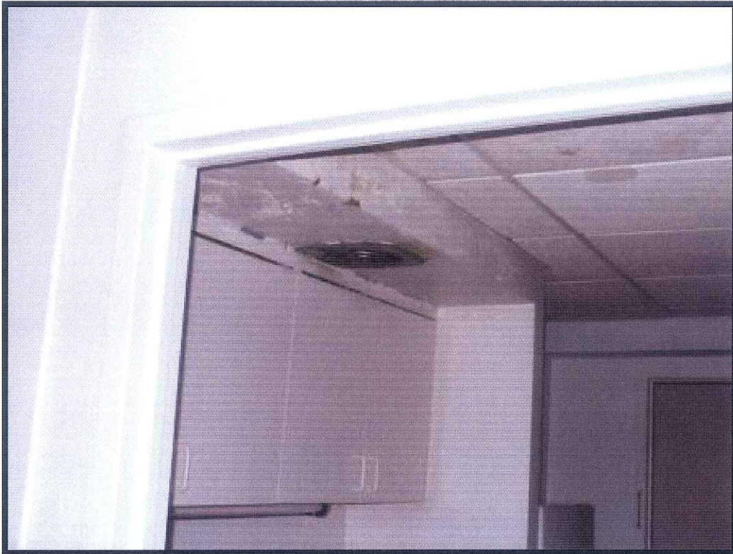
Water damage in kitchenette
