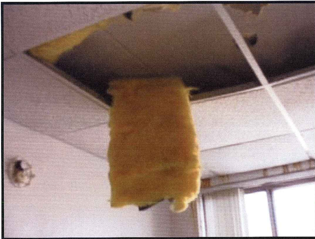
Additional water damage from leaking roof
