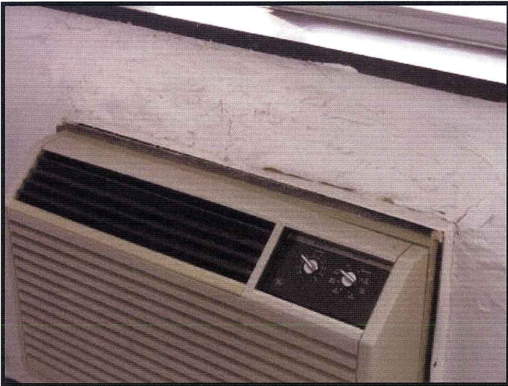
Apartment air conditioner
