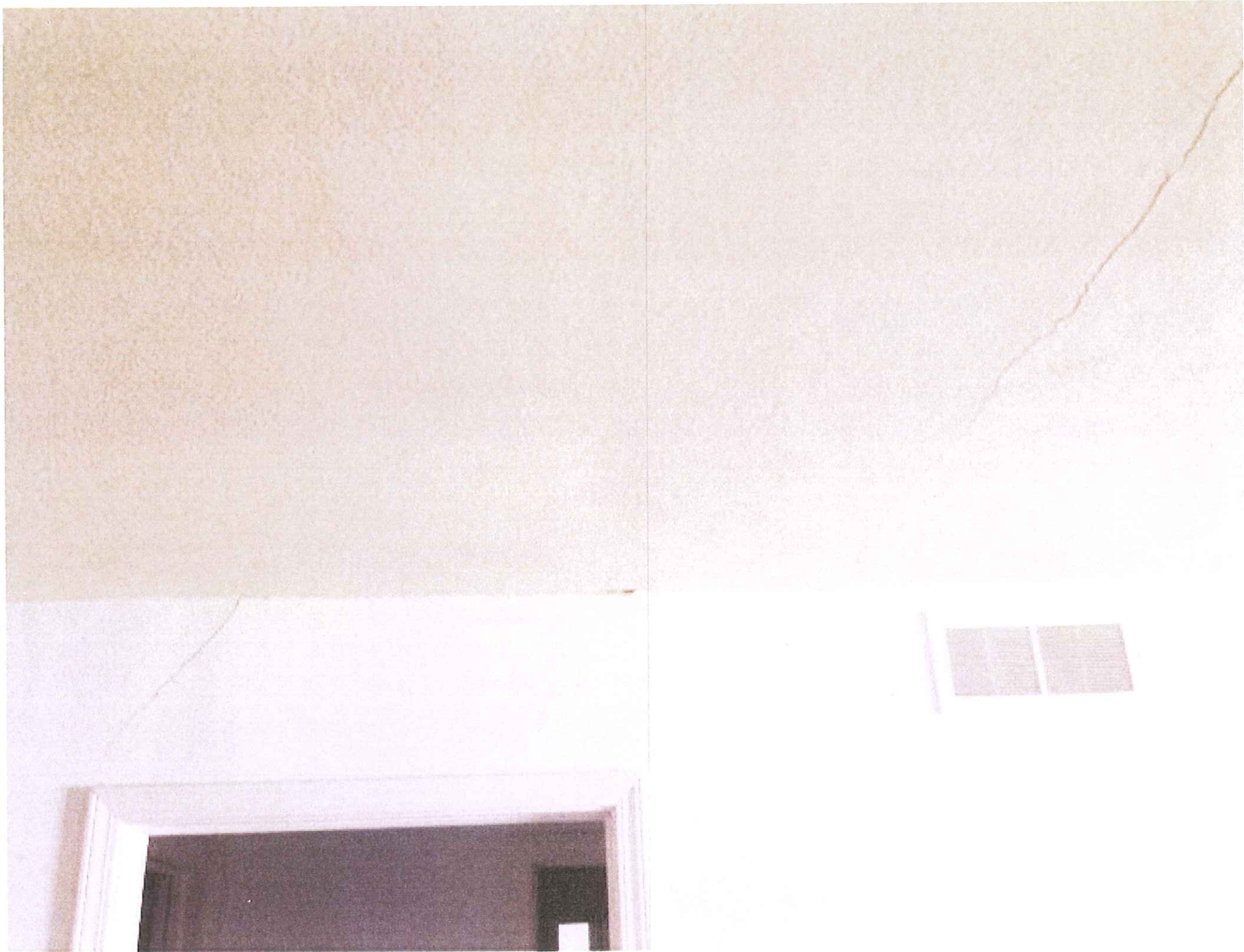
MANY CRACKS - FROM ABNORMAL SETTLING AND SHRINKING
