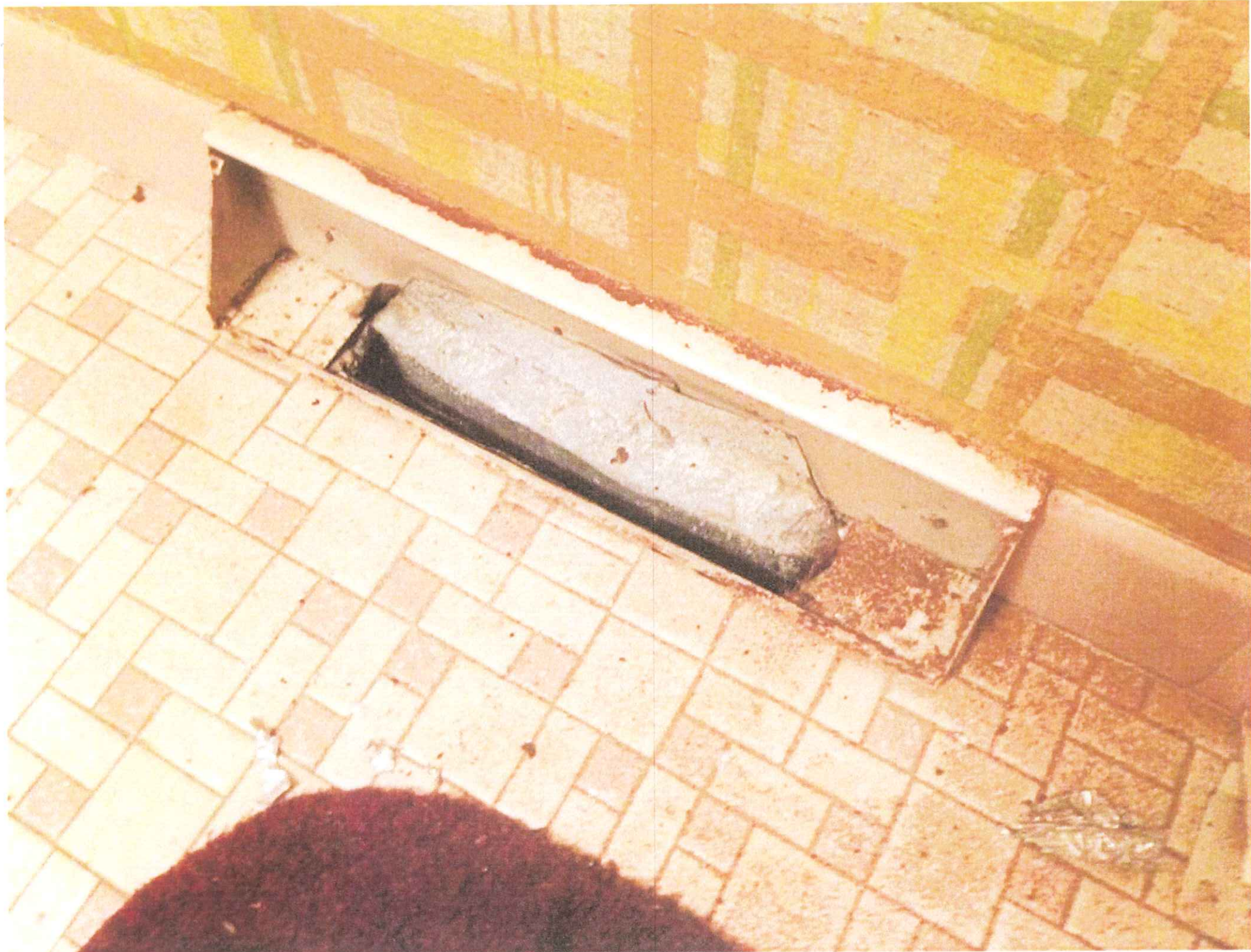
L.L. DUCT COMING OUT OF FLOOR - RUST-MOLD CAUSED BY WATER UNDER SLAB
