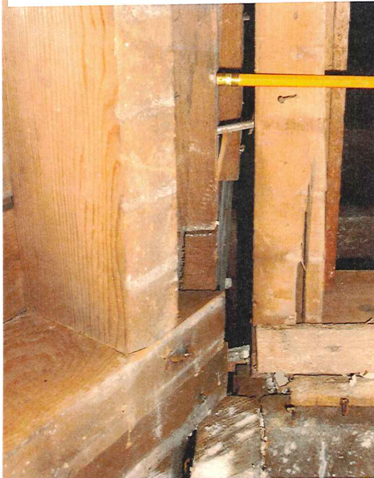
2 Interior NE corner wall separation @ 1st Floor 214 S Marquette Street
