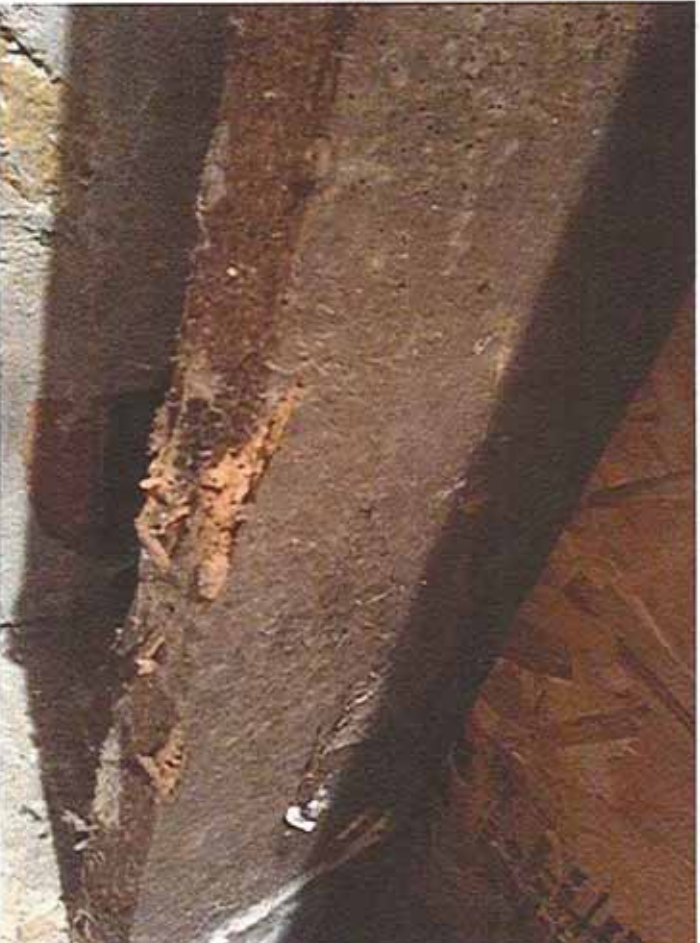
Image 26: Floor joist with apparent insect deterioration.
