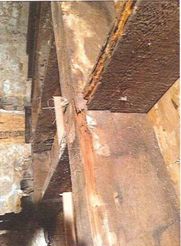
Image 16: Floor joist with apparent insect deterioration.
