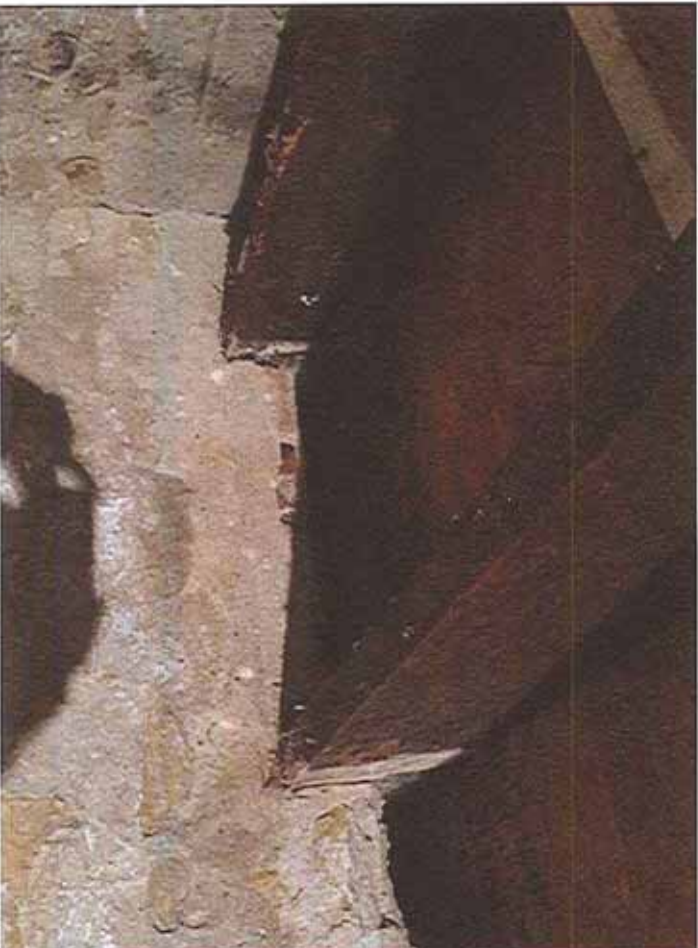
Image 25: Joists bearing directly on concrete foundation wall.
