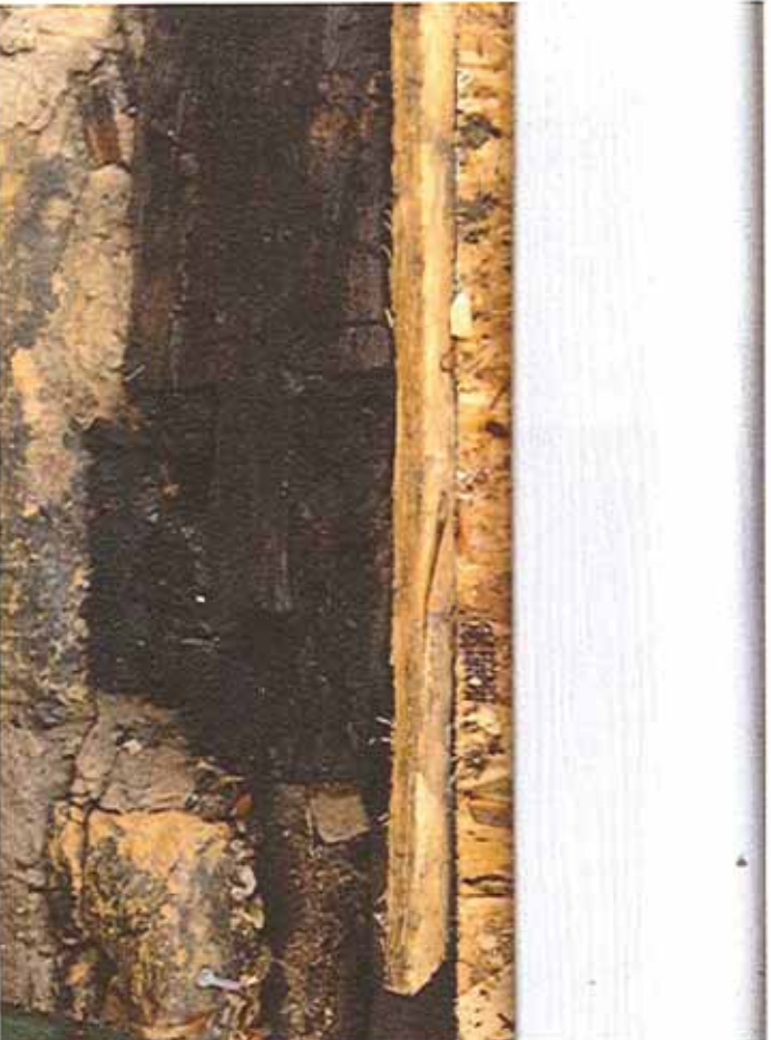
Image 8: Rotting wood bearing on the foundation wall.
