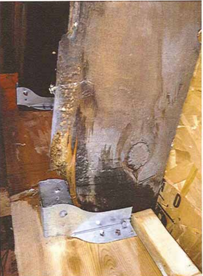
Image 12: Deteriorated joist with new clip.
