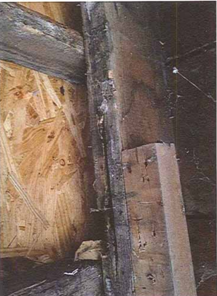
Image 41: Deteriorated framing at exterior wall.
