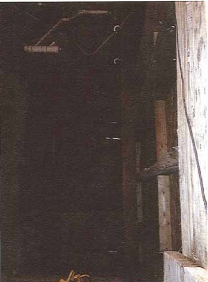
Image 28: View of undersized support beam.
