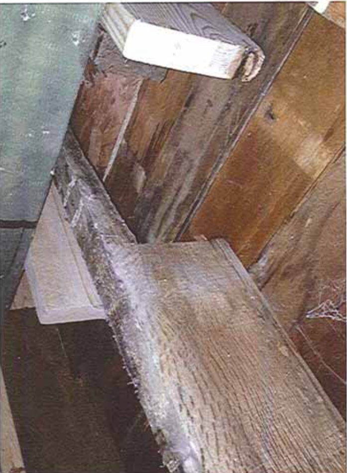
Image 17: Floor joist with notch bearing on support beam.
