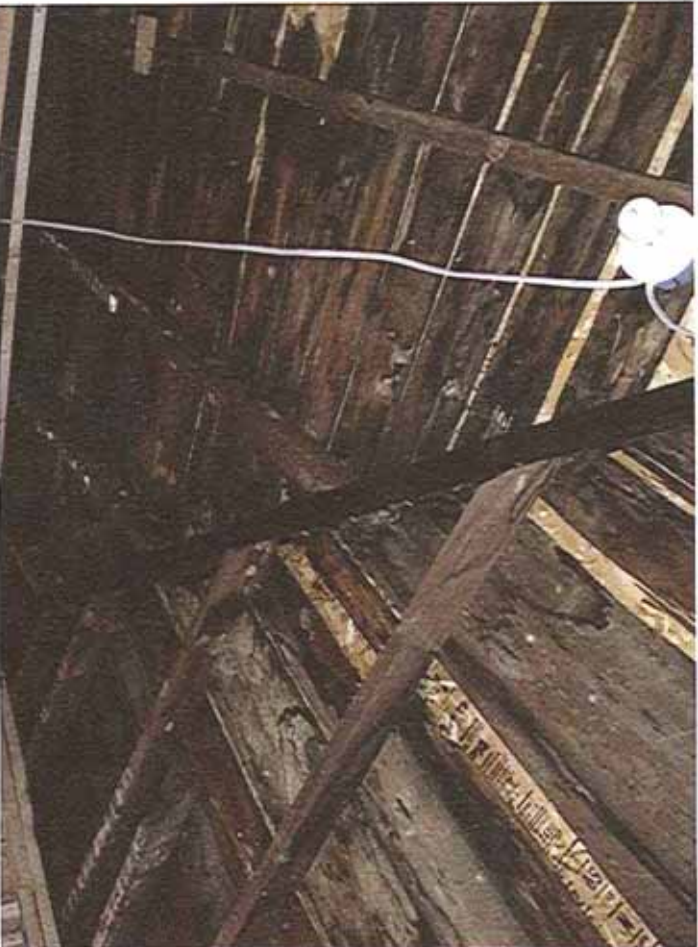
Image 32: Undersized hip beam.
