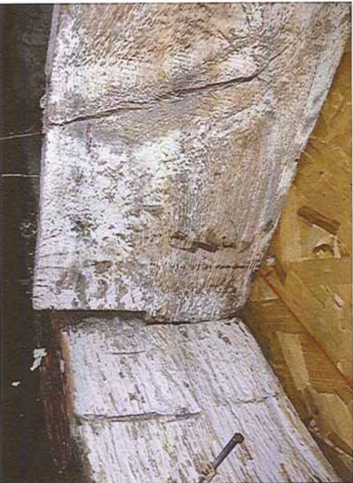
Image 31: Floor joist with notch exceeding NDS limitations.
