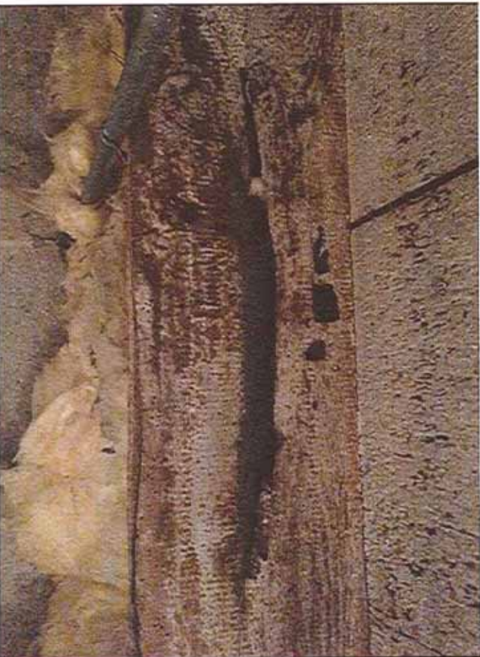
Image 27: Floor joist with damage/deterioration.
