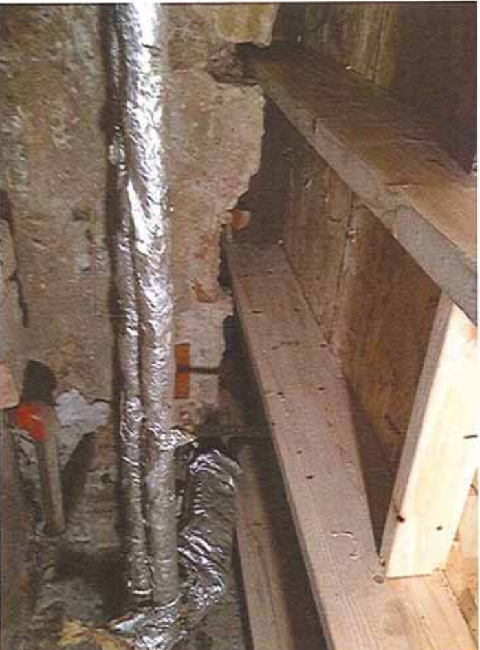
Image 14: New floor joists not bearing on foundation wall, supported by rim joist.
