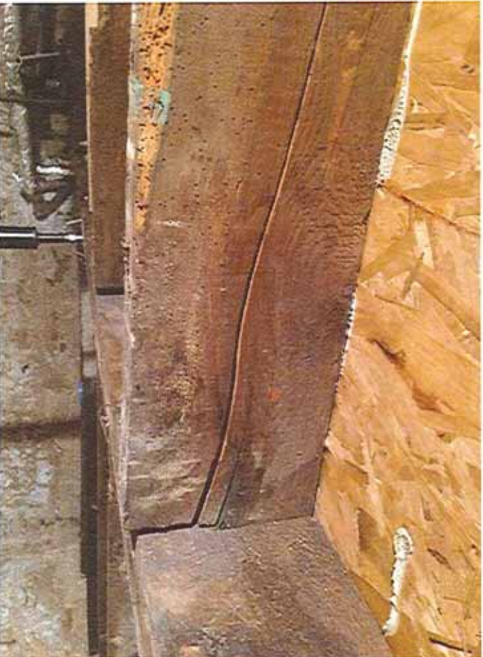
Image 22: Joist with apparent insect deterioration and shear failure.
