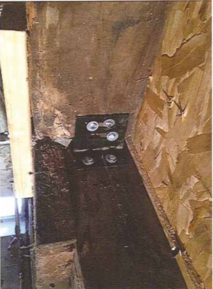
Image 24: Beam to beam connection. Note deterioration.
