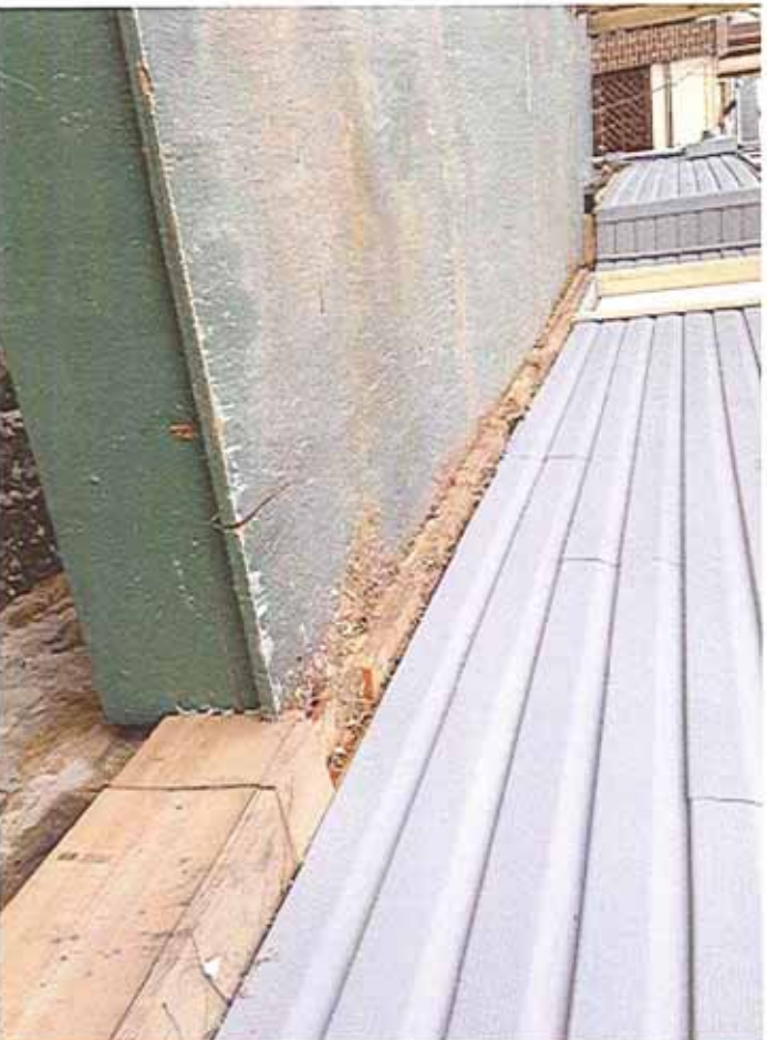
Image 7: First floor framing extending beyond the face of the foundation wall & exterior wall framing.
