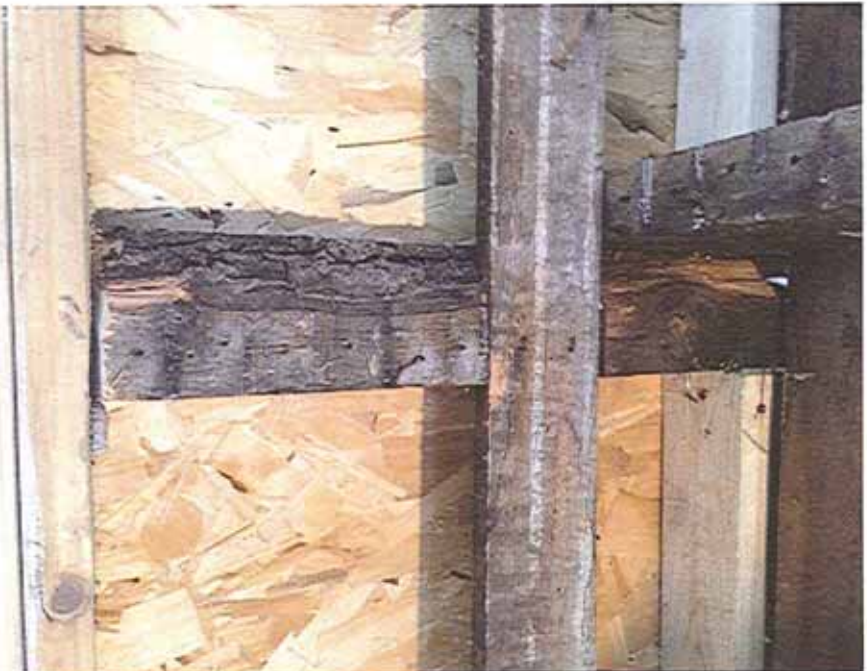
Image 38: Deteriorated wall stud.
