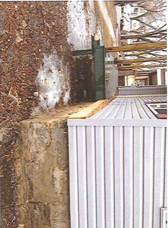
Image 6: First floor framing extending beyond the face of the foundation wall & exterior wall framing.
