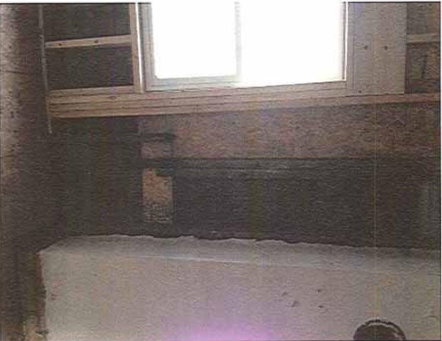
Image 39: Discontinuous wall stud.
