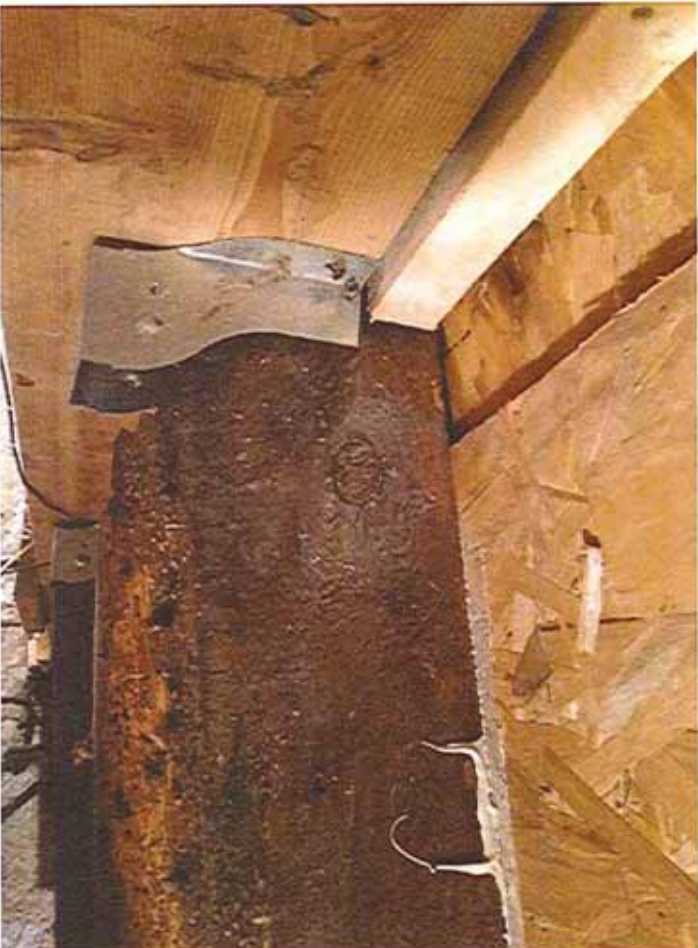
Image 21: Joist with apparent insect deterioration.
