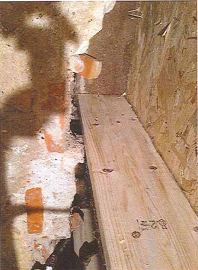
Image 15: New floor joists not bearing on foundation wall, supported by rim joist.
