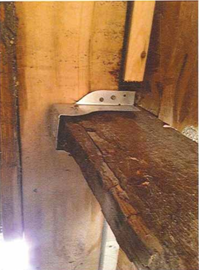
Image 23: Joist with deterioration and new hanger.
