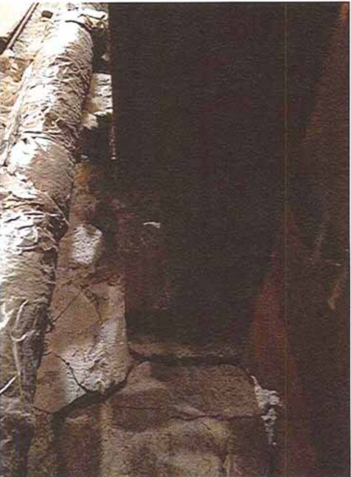
Image 11: Wood beam bearing directly on concrete with notch.
