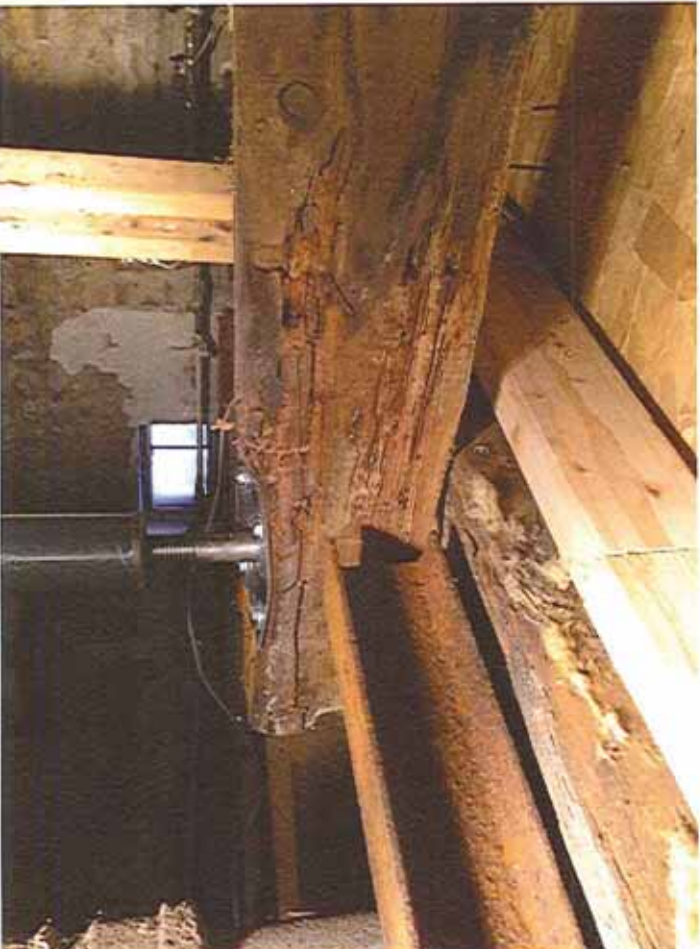
Image 13: Severely deteriorated support beam.
