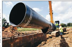
A section of water main is lowered into a trench by Jeff McGee, holding pipe, and Dave Hill, working along together in Fitchburg. Development in cities such as Fitchburg and Verona is a threat to the state's aquifer system. But the demand has led to increased impacts on surface waters such as wetlands and streams.
