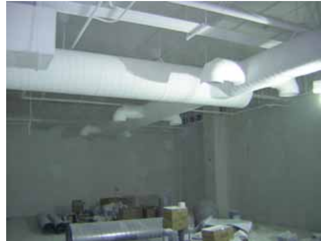
Picture above shows new painted ceilings and exposed duct work in one of the new basement rooms.
