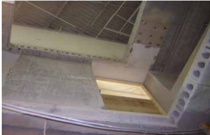
Picture above shows the new elevator shaft. Crews have just finished cutting the slab openings.
